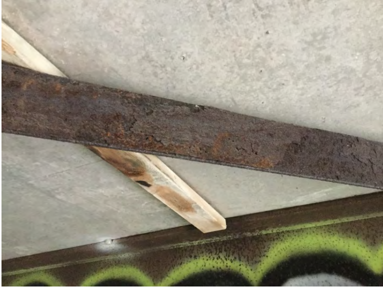
Minor steel delamination on plan bracing
