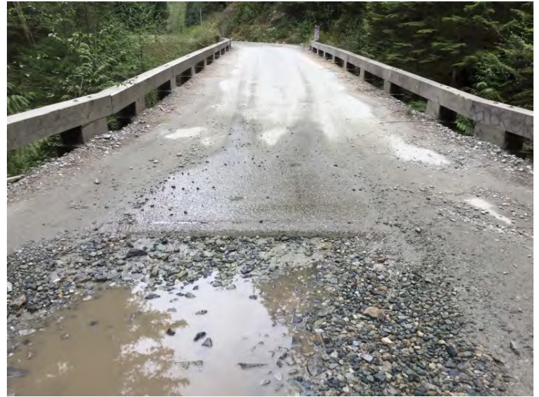
Potholes at left approach
