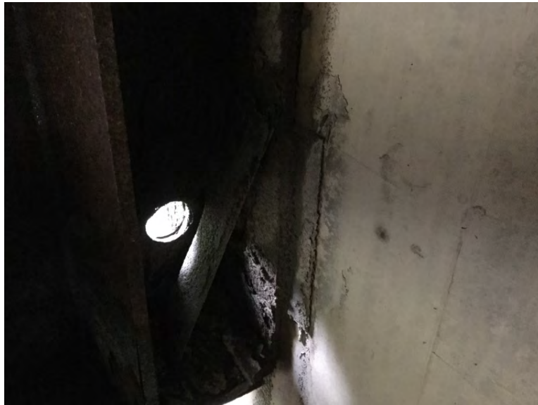
Minor steel delamination of end plates
