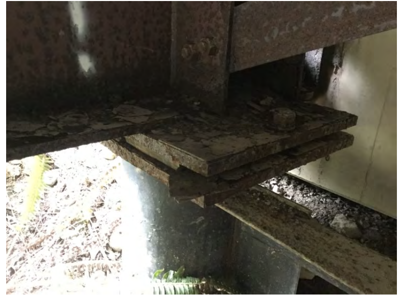
Minor delamination of bearing plates and bottom flange around bearing locations
